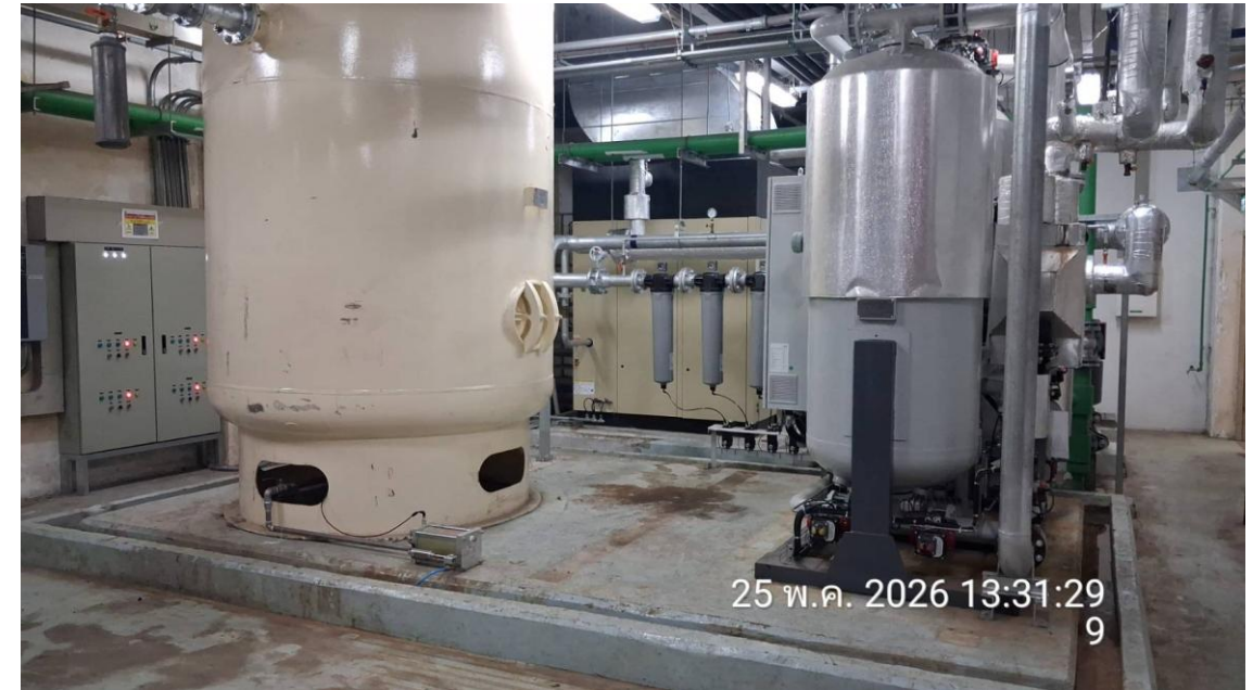
Compressed Air Receiver Tank & Adsorption Dryer
